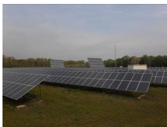
Photovoltaikanlage in Zwentendorf
